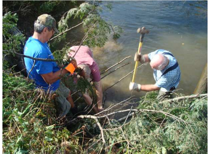
Volunteers hammer in anchor and cable to hold tree revetment in place
