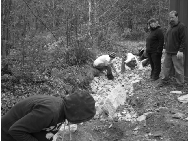
Students from Richford Highschool helped stone-line a ditch along Creamery Bridge Road in Montgomery last fall.
